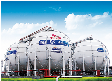
Cryogenic Liquid Spherical Storage Tanks
