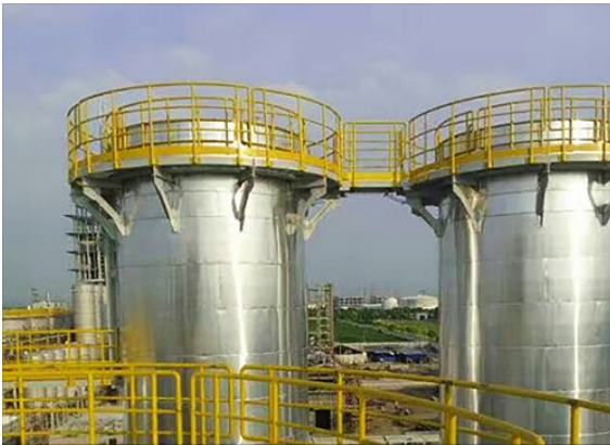
Grease Storage Tanks
