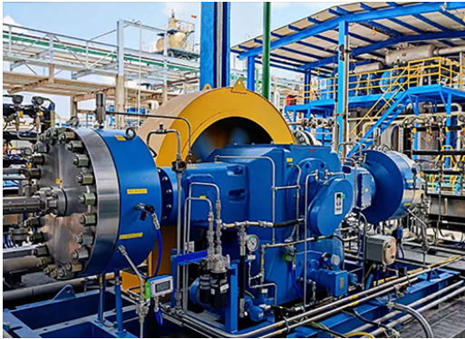
Hydrogen Refueling Mother Station
